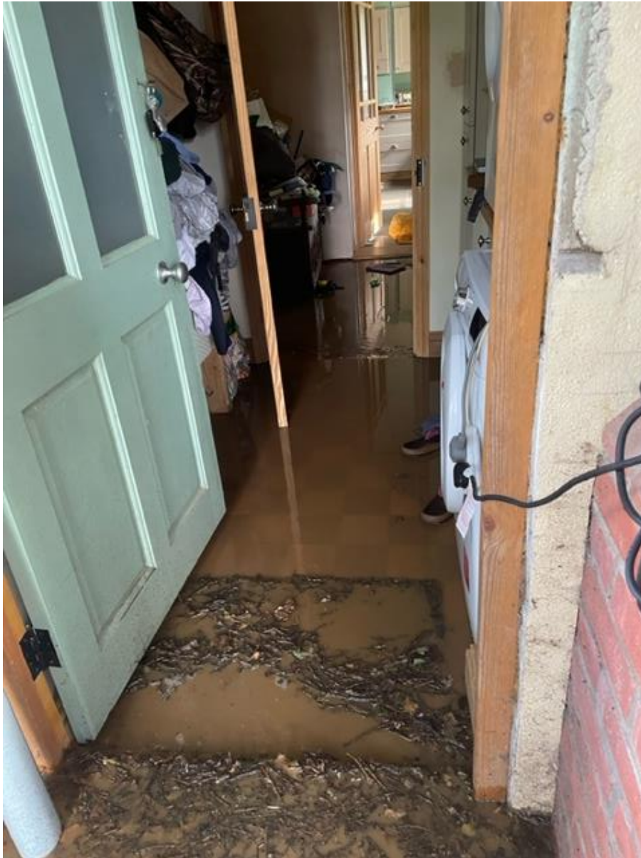
Photo 1 – Internal flooding photograph provided by resident in August 2023.
