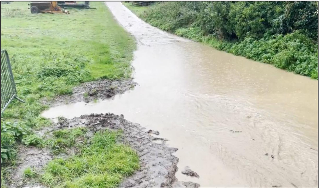
Image 5 - Surface water runoff from Witten's Meadow construction site towards Mow Hill (photo looking southwest)
