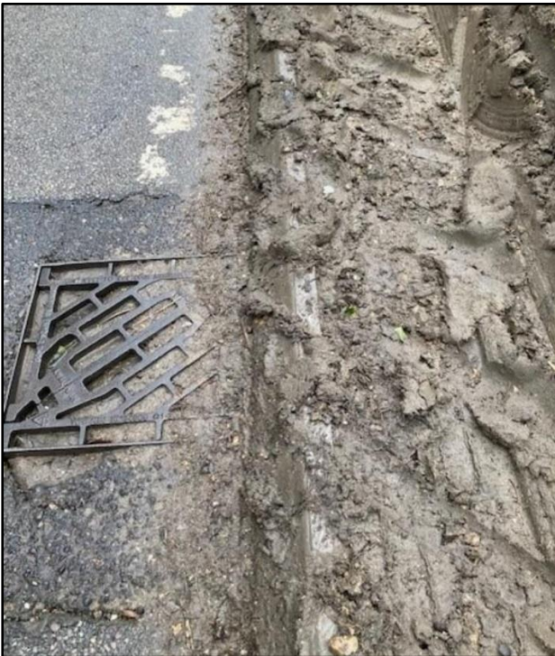
Image 7. Gully on Swan Hill, A1120, blocked by erosion of verge
