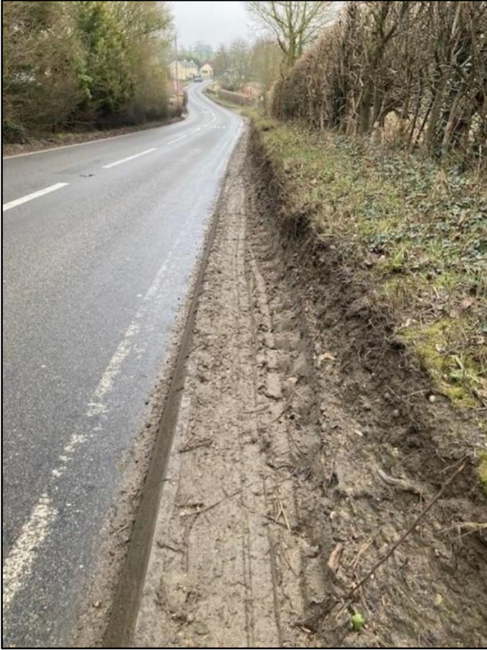
Image 6. View down Swan Hill, A1120, showing erosion of verge
