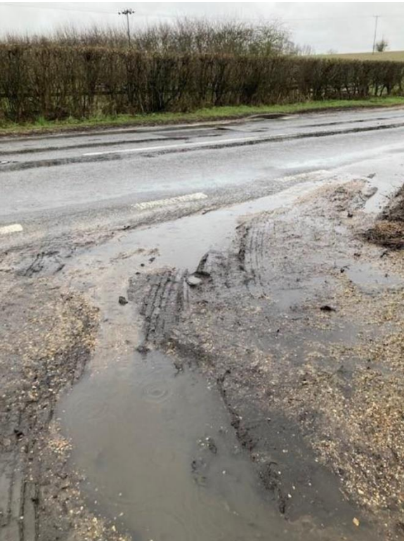
Image 5. Surface water pathway from the A1120 on to property at the bottom of Swan Hill
