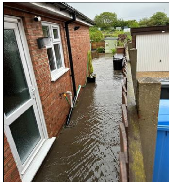
Flood water flowing from Ashcroft Road to the back garden of property B
