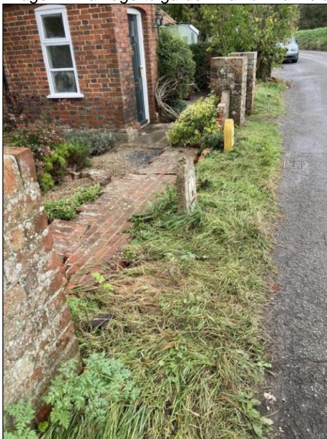
Image 7 - Damage to garden wall on Fairfield Road
