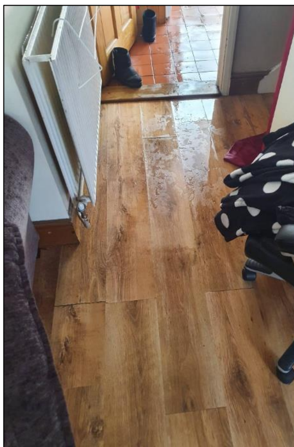
Floodwater accumulating inside the kitchen and living room of one of the flooded properties
