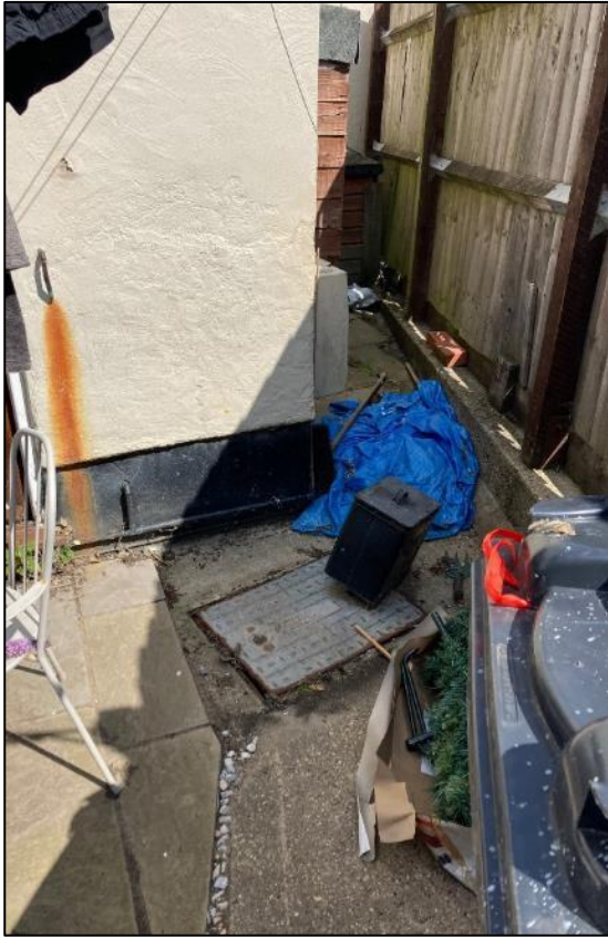
Manhole (foul sewer) in the rear garden that had recently surcharged
