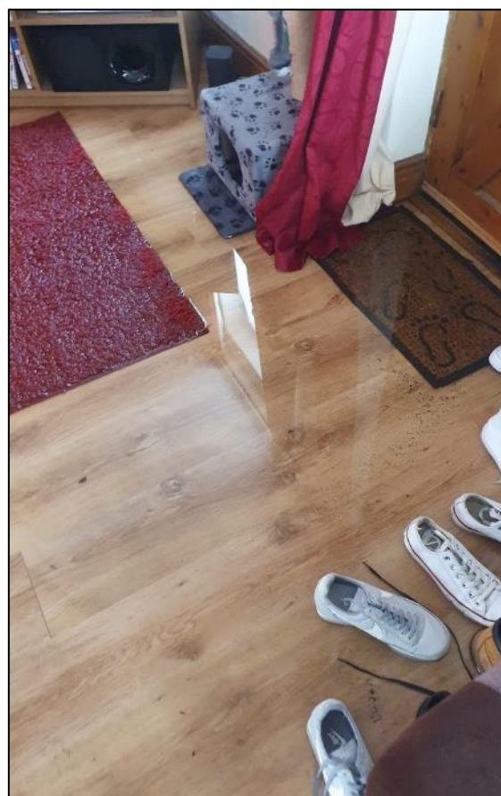
Floodwater accumulating inside the living room of one of the flooded properties
