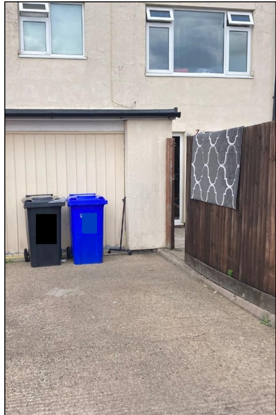
Access gate through fence where surface water travelled into property from the rear
