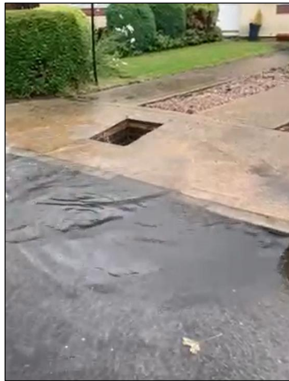
Surface water accumulating in the highway outside Property A, Elm Close.
