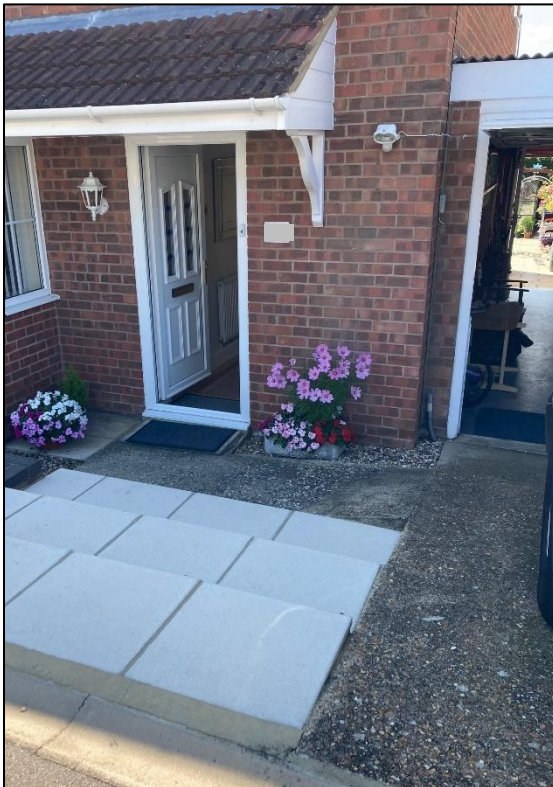
Sloped driveway/steps down from highway towards Property C, Greenwood Close directing runoff into the front of the house
