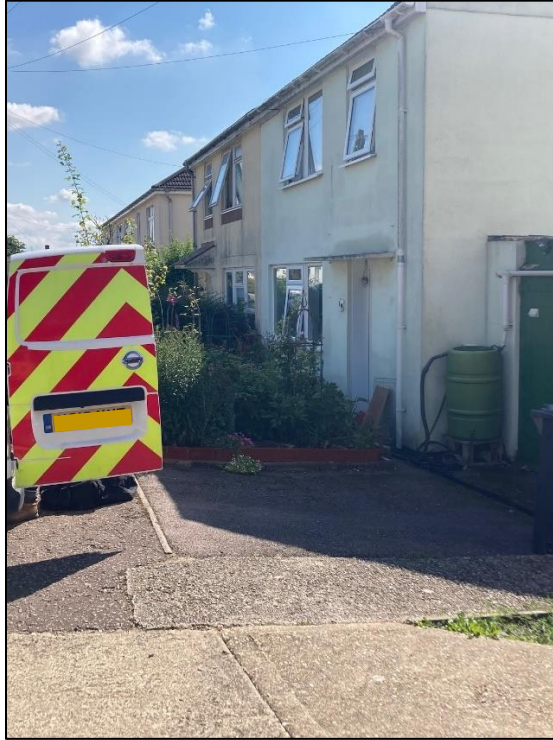
Slope down from highway towards Property B, Hazel Close directing runoff into the front of the house
