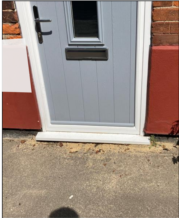
Depth of flooding externally, water reported to have reached lower edge of the letter box
