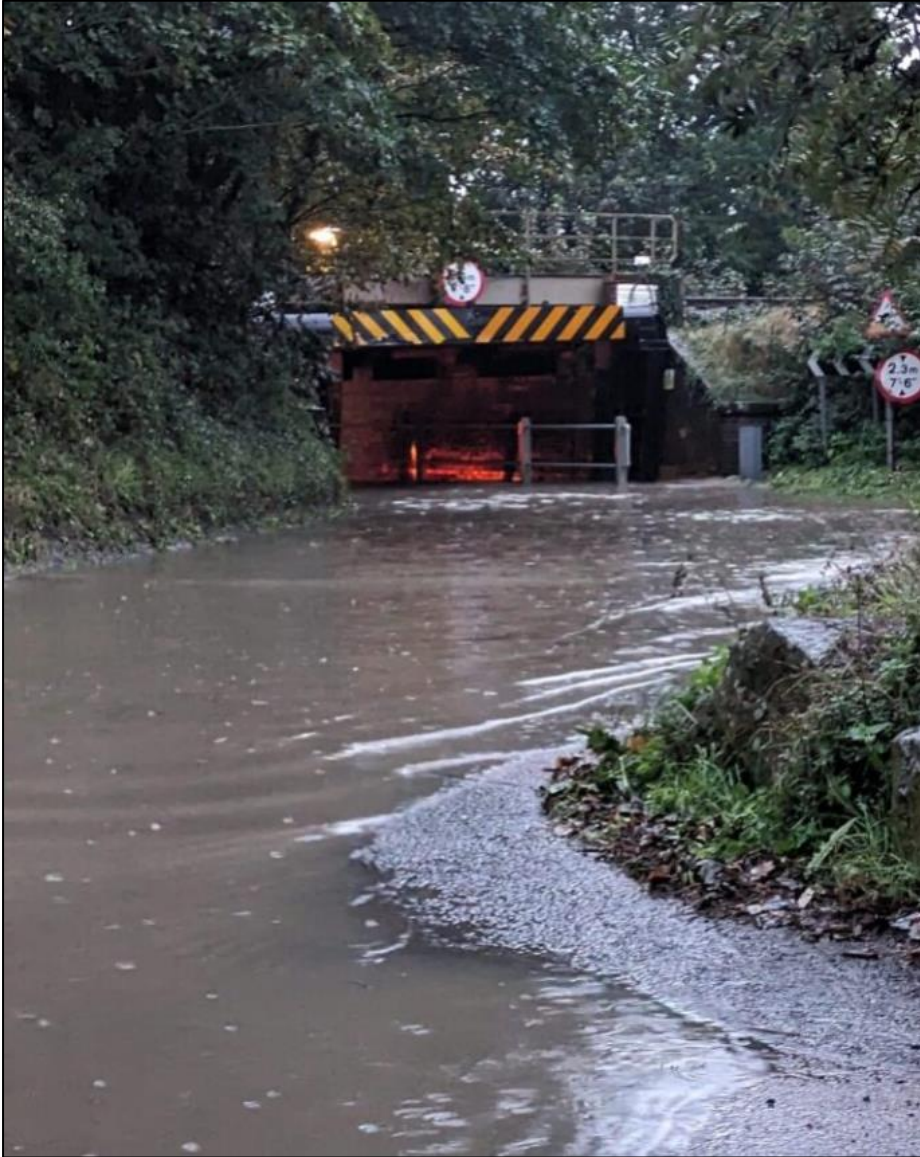
Image 7 - Flooding under Coddanham Road railway bridge
