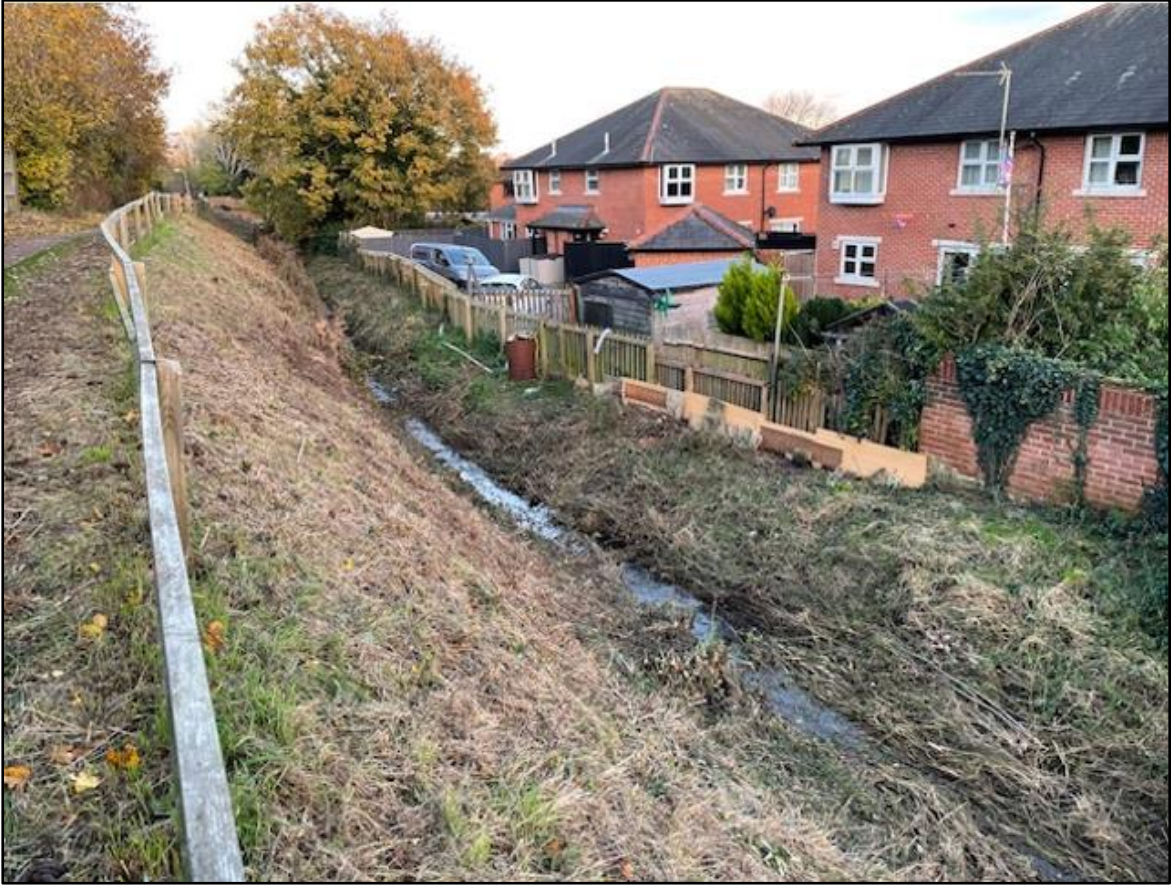
Image 10 - Makeshift defences against floodwater overtopping from Orchard Gate watercourse
