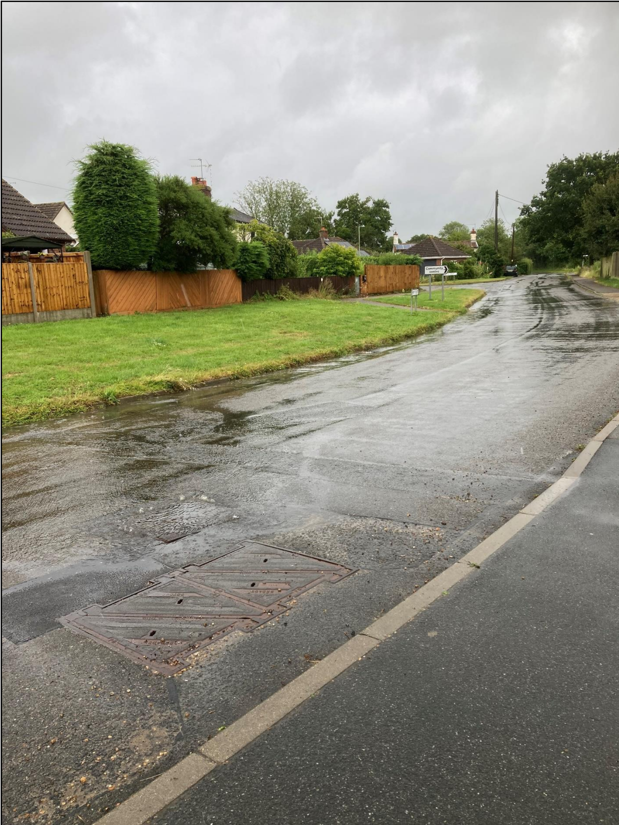
Image of the Sewerage network being overwhelmed by surface water (not taken during Babet)
