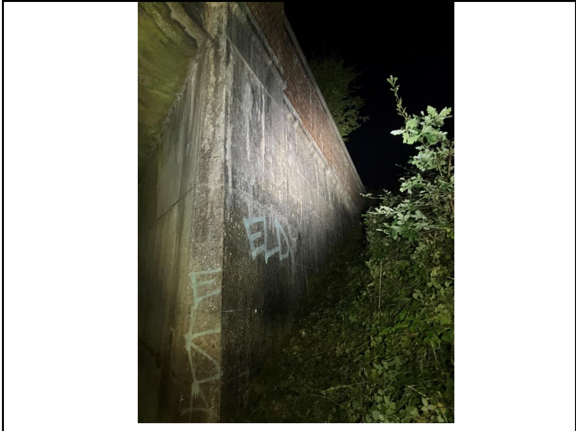
1717_P53_2024 Northwest wingwall – Saline leaching
