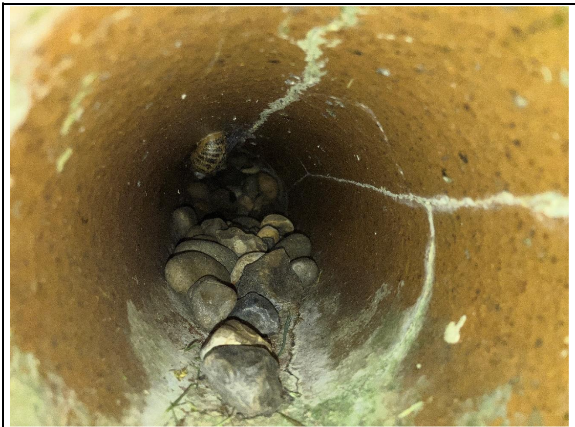
1717_P27_2024 West abutment - Weep hole partially blocked
