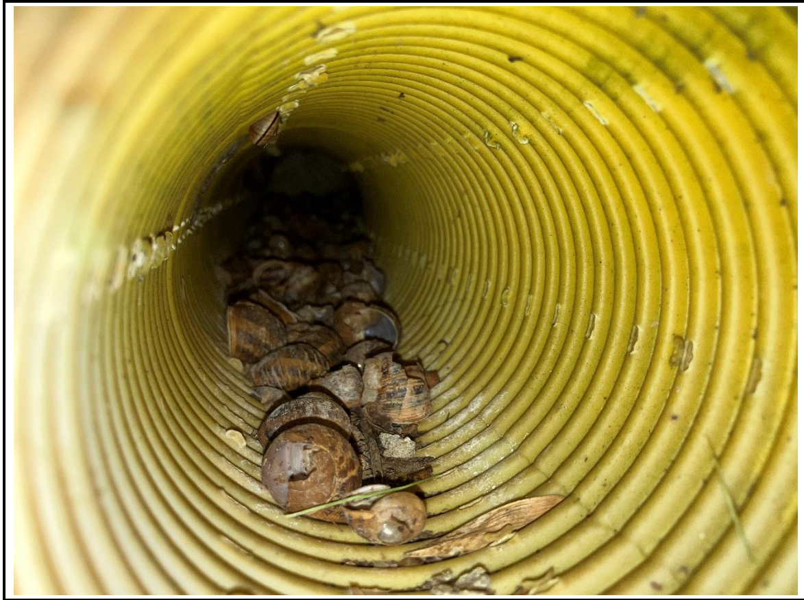
1717_P28_2024 Southeast wingwall - Weephole partially blocked
