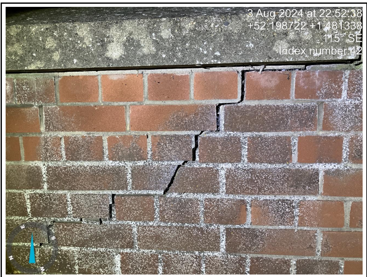
1717_P33_2024 South parapet - Diagonal parapet crack (<10mm)
