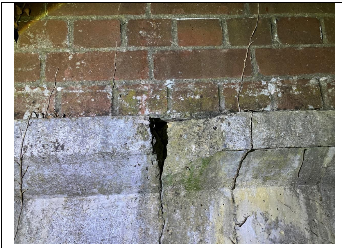
1717_P46_2024 Southwest wingwall - Concrete spalling & Vertical crack
