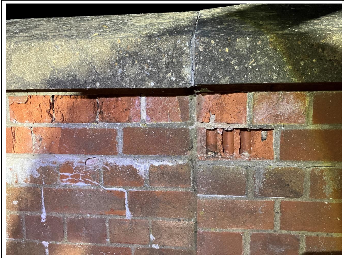
1717_P40_2024 North parapet - Brick spalling & hairline cracks
