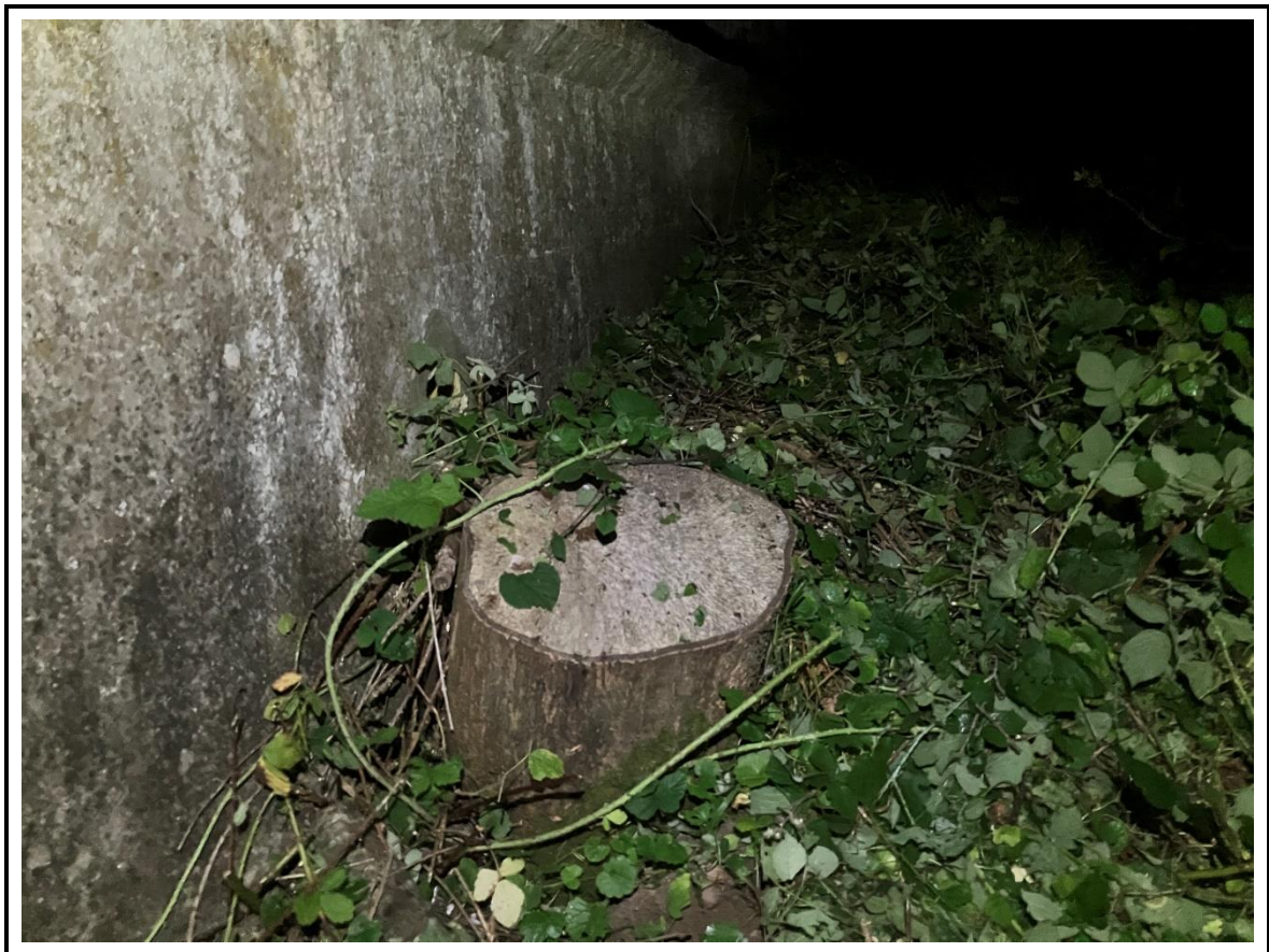
1717_P56_2024 Northwest wingwall - Vegetation growth
