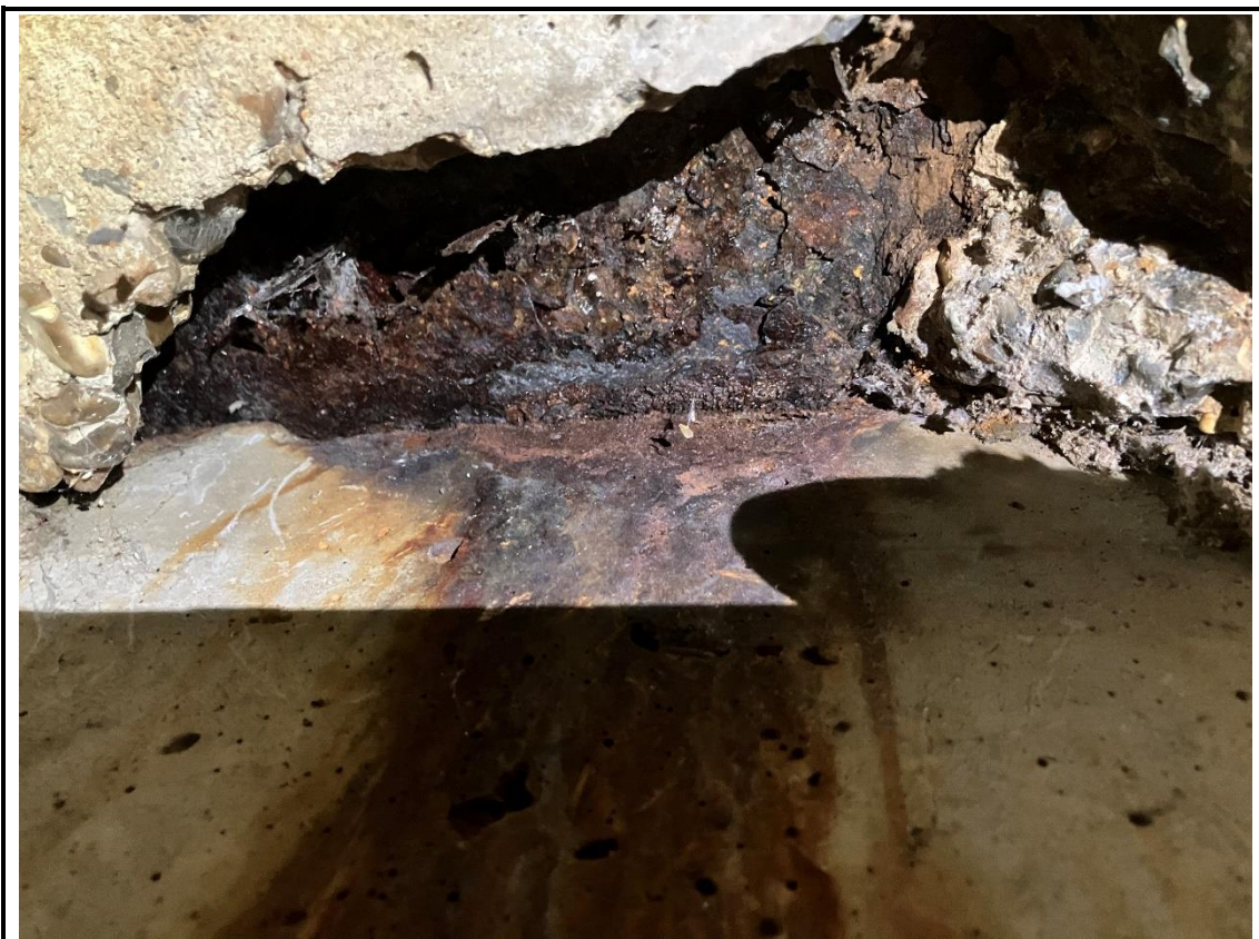
1717_P6_2024 West abutment/soffit interface - Exposed steel beam flaking corrosion
