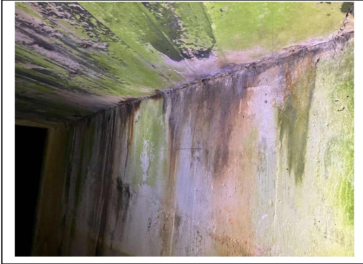
1717_P23_2024 East abutment - Saline leaching and corrosion staining
