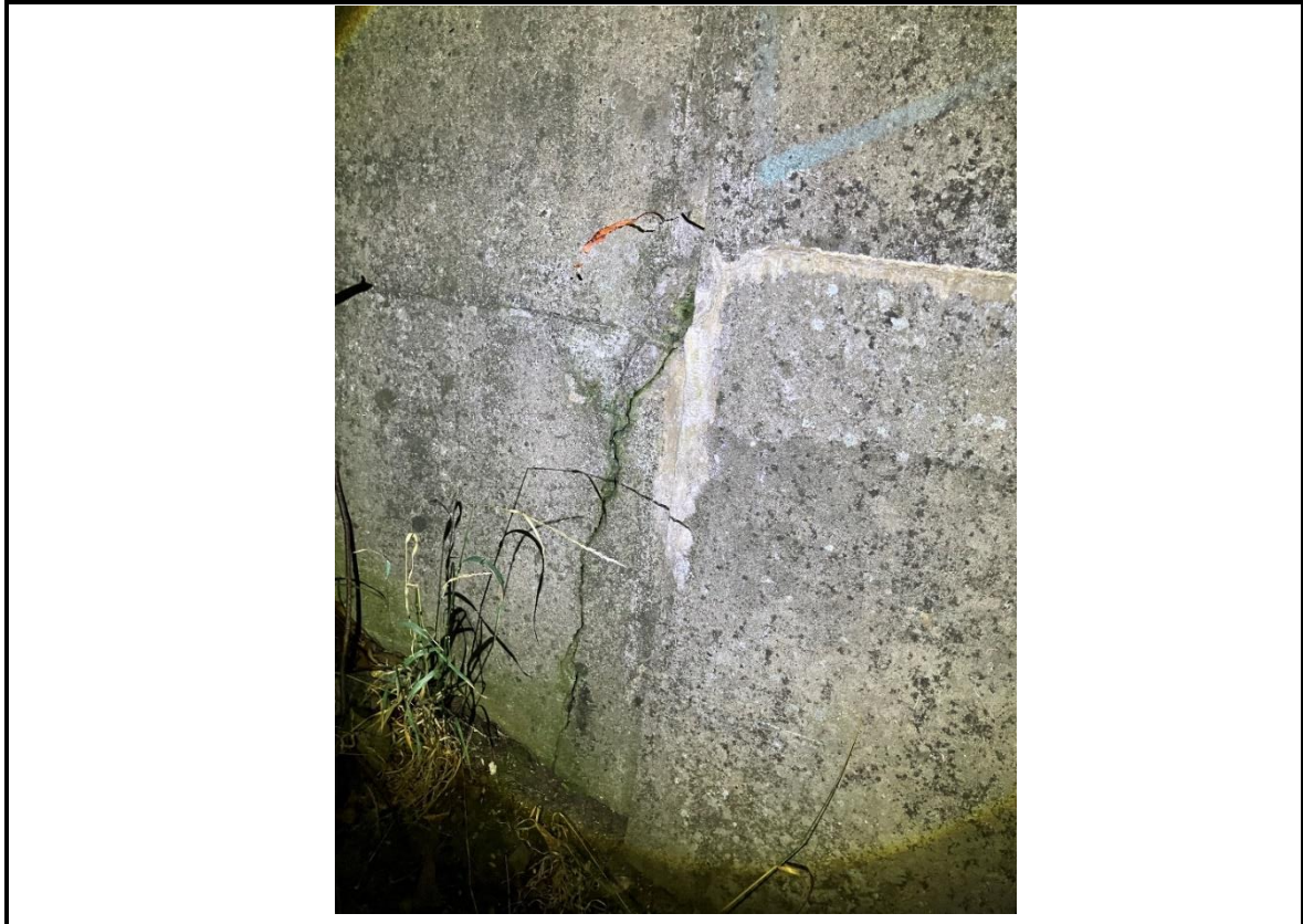
1717_P47_2024 Southwest wingwall/abutment - Concrete spalling & diagonal crack
