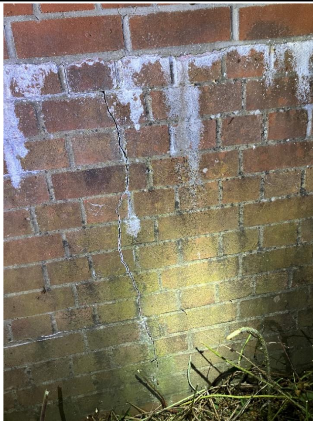
1717_P39_2024 North parapet - Vertical Crack (<1.5mm) & leaching
