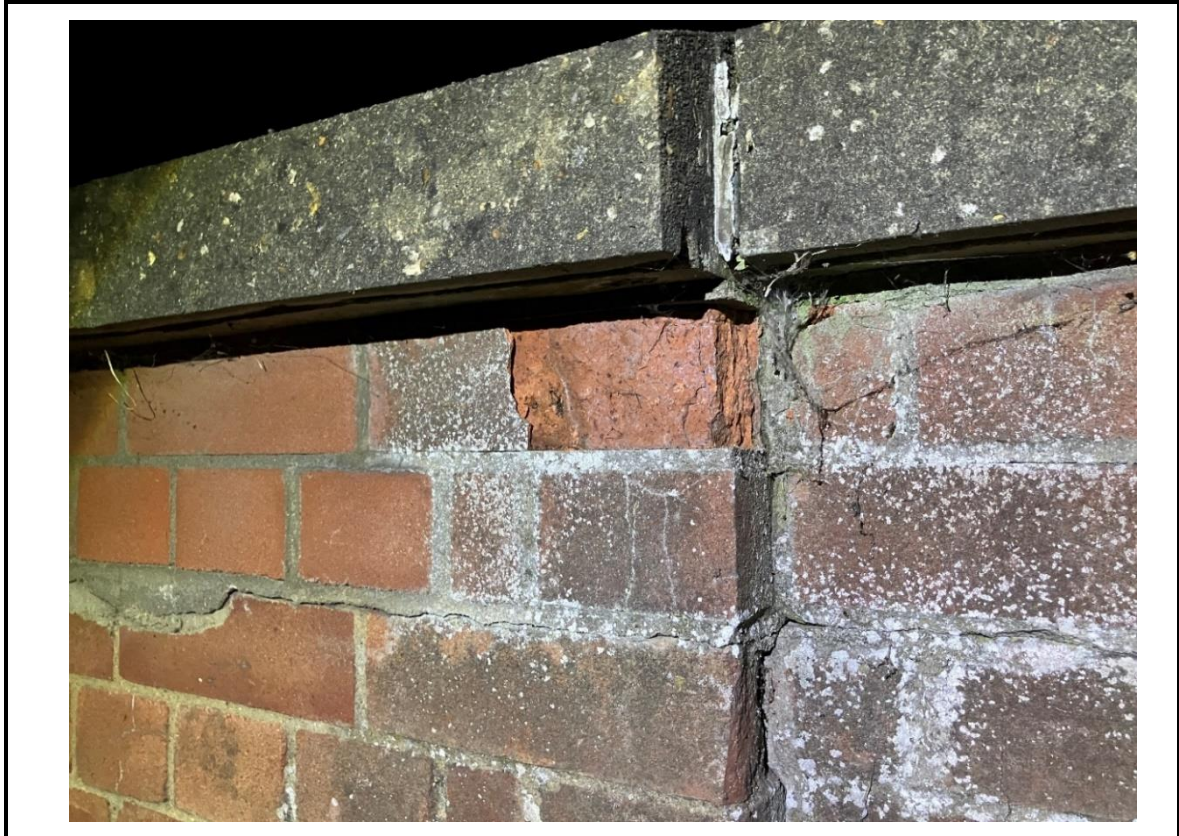
1717_P34_2024 South parapet - Brick spalling (10mm deep) & horizontal hairline crack
