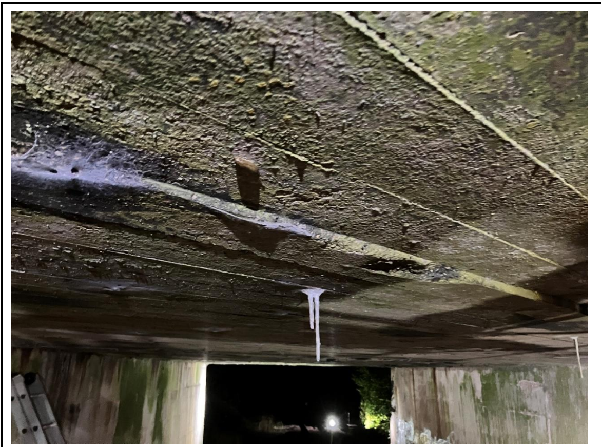
1717_P31_2024 Bridge soffit - Stalactite formation (<150mm)
