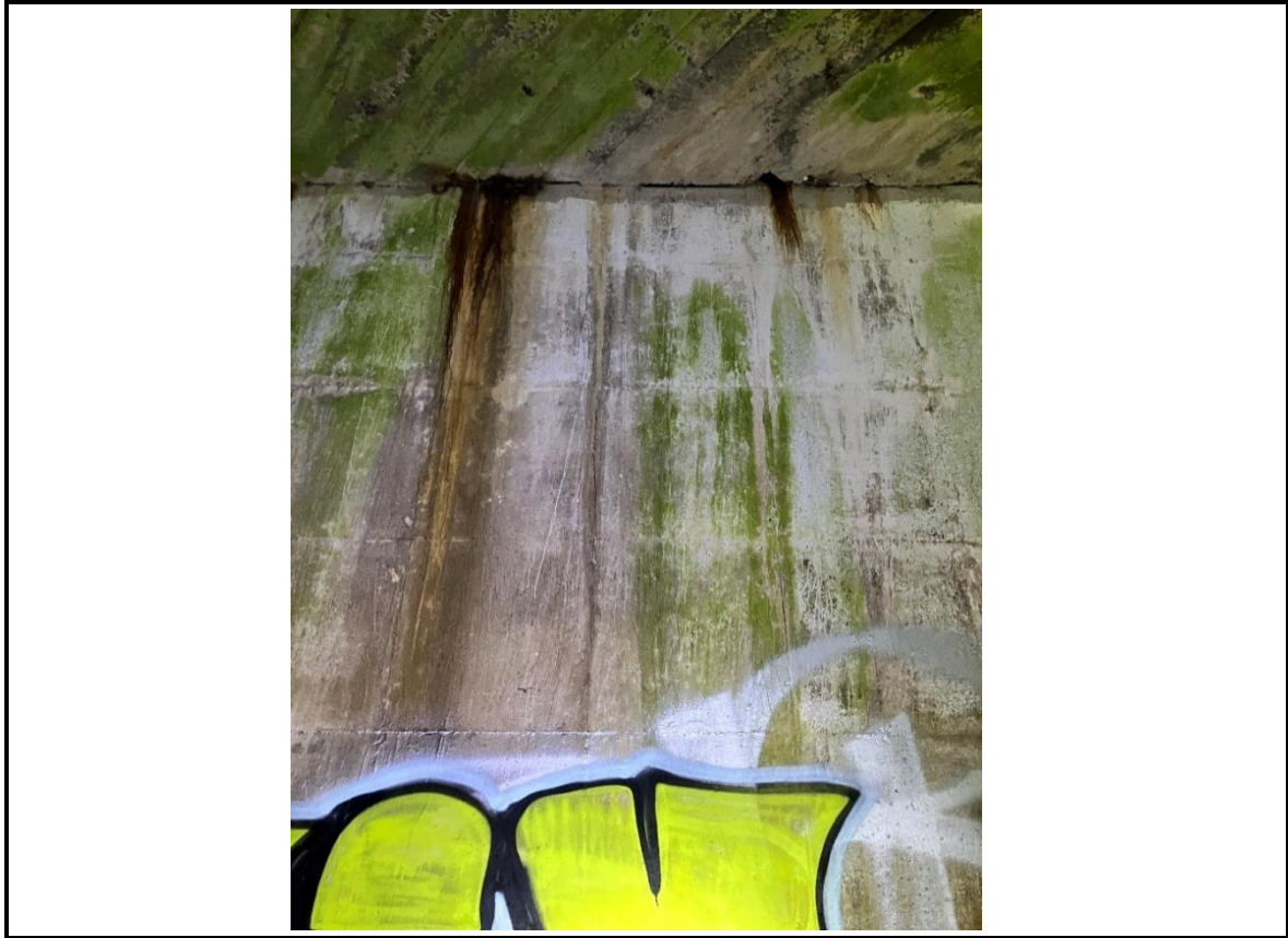
1717_P19_2024 West abutment - Saline leaching and corrosion staining
