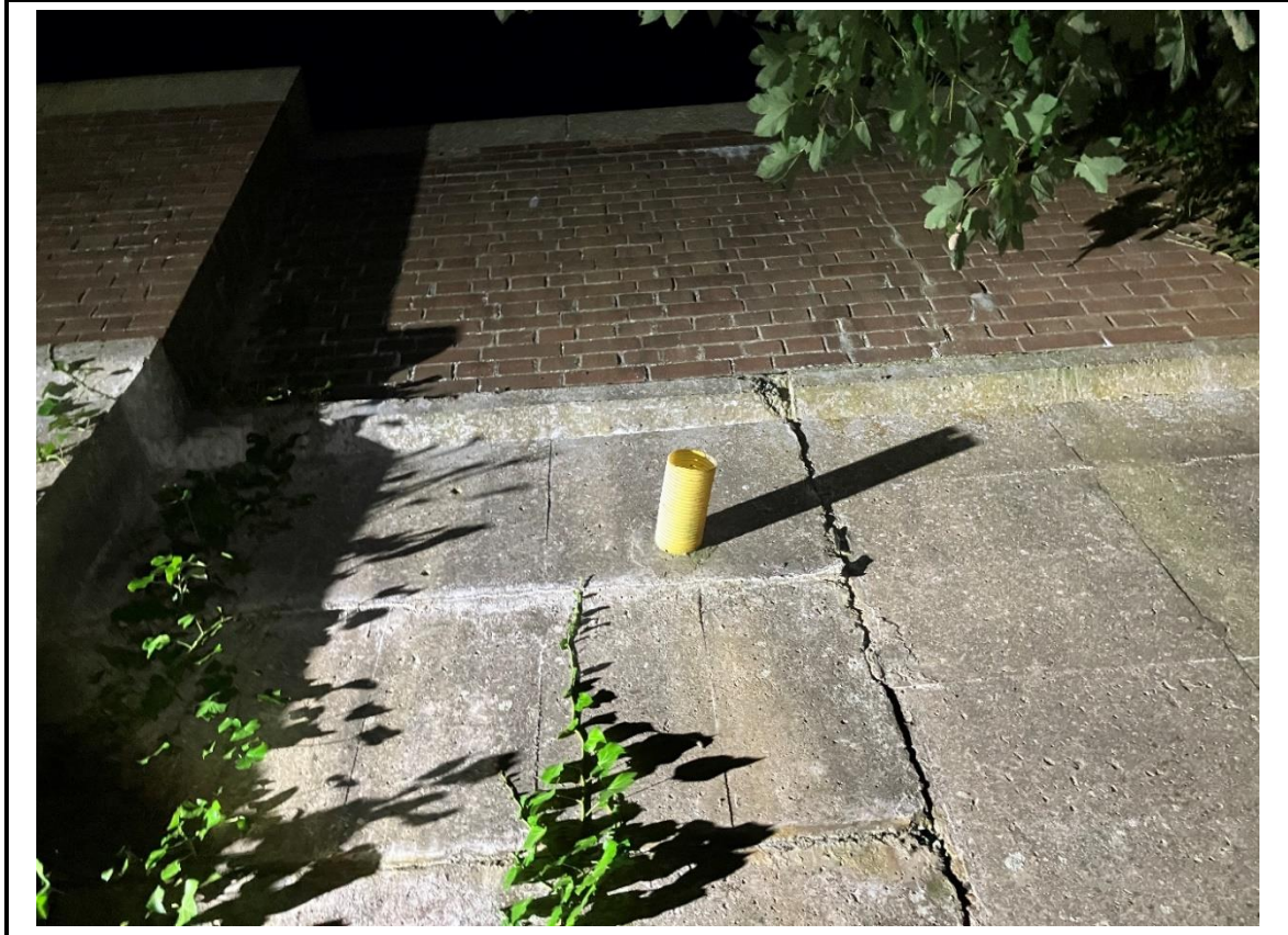
1717_P51_2024 Southeast wingwall - Vertical cracking (<3.5mm) & minor spalling
