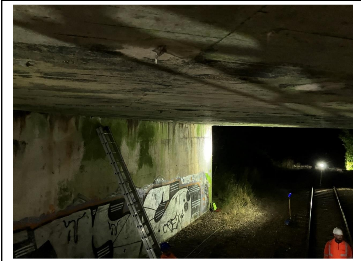
1717_P21_2024 East abutment - Saline leaching, corrosion staining and graffiti
