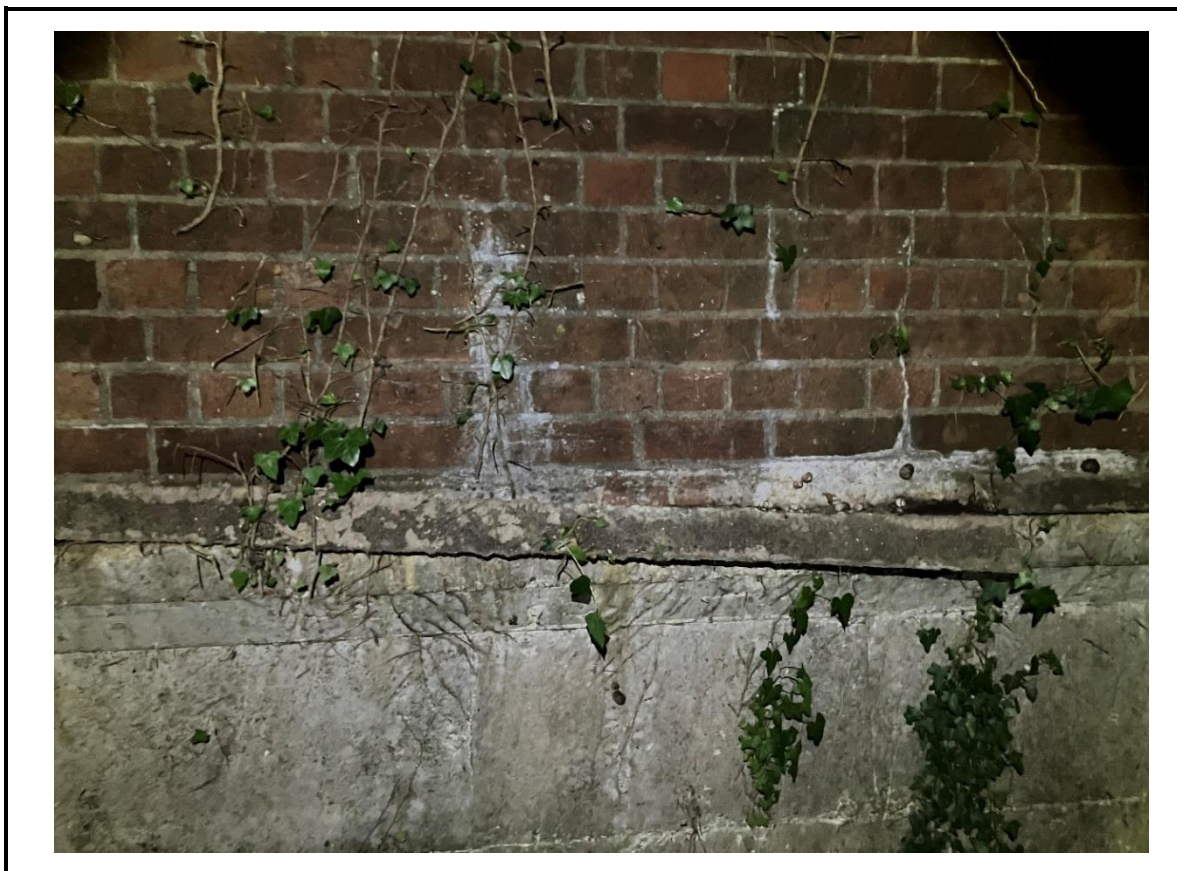
1717_P50_2024 Southeast wingwall - Mortar fillet peeling off
