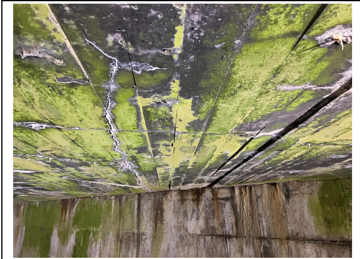
1717_P22_2024 East abutment - Saline leaching and corrosion staining
