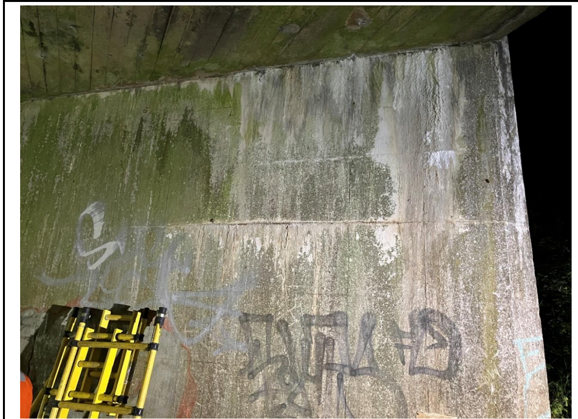
1717_P18_2024 West Abutment – Saline leaching (<30mm at the top)
