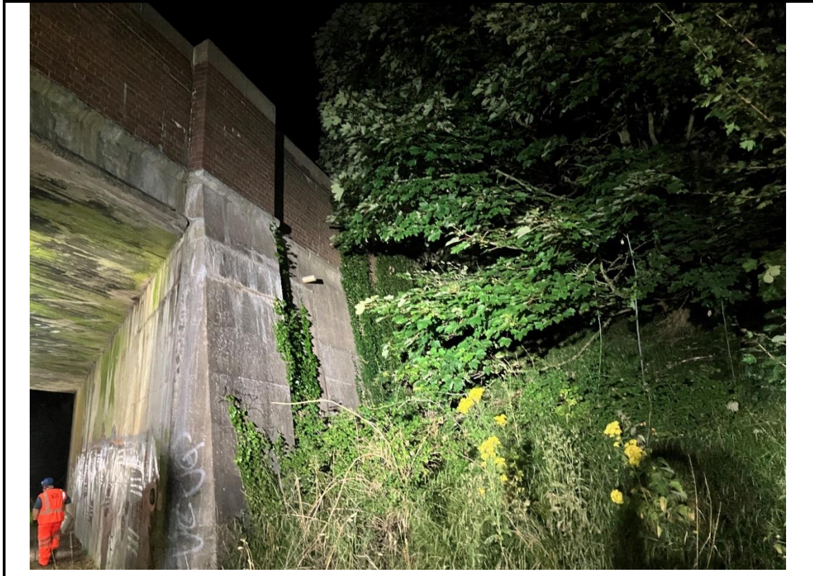
1717_P49_2024 Southeast wingwall – Saline leaching & vegetation growth
