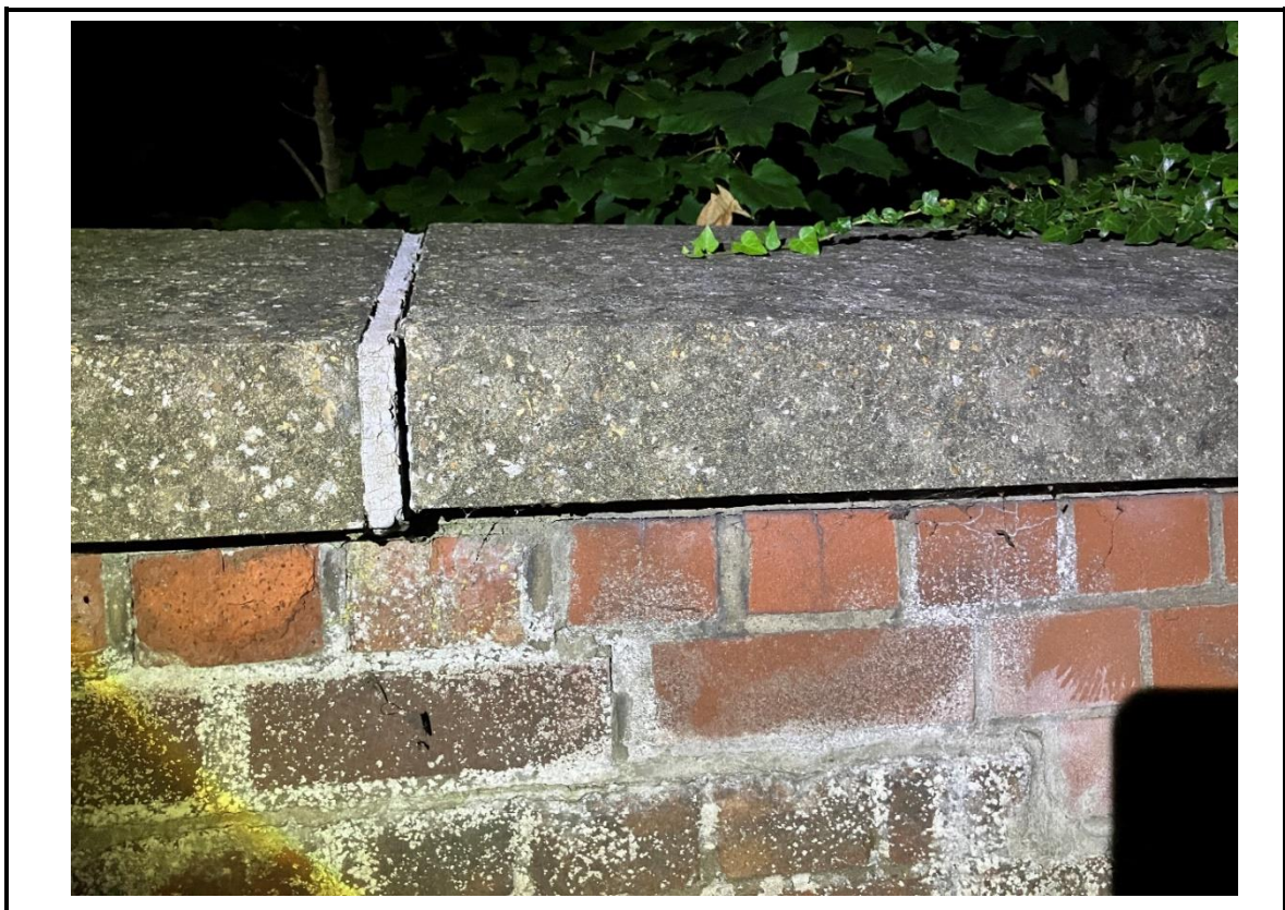
1717_P35_2024 South parapet – Displacement of parapet coping (<15mm) & repaired diagonal crack
