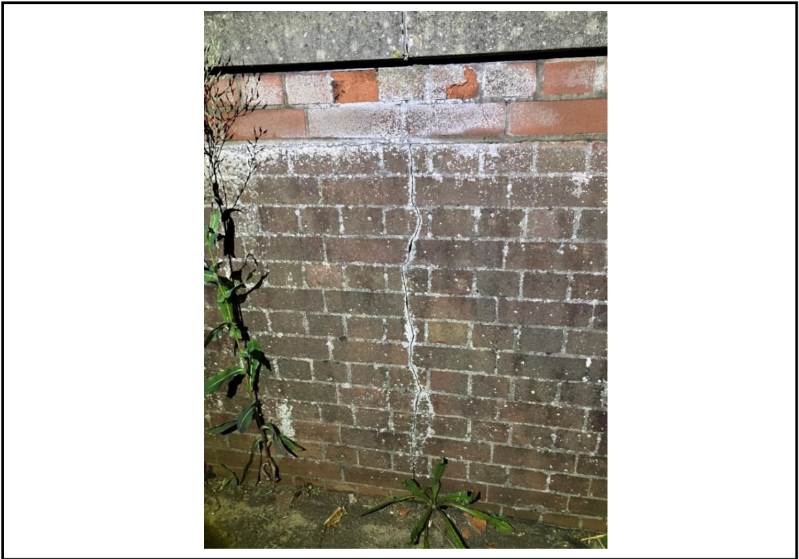
1717_P32_2024 South parapet - Vertical and hairline horizontal cracks (<2mm)
