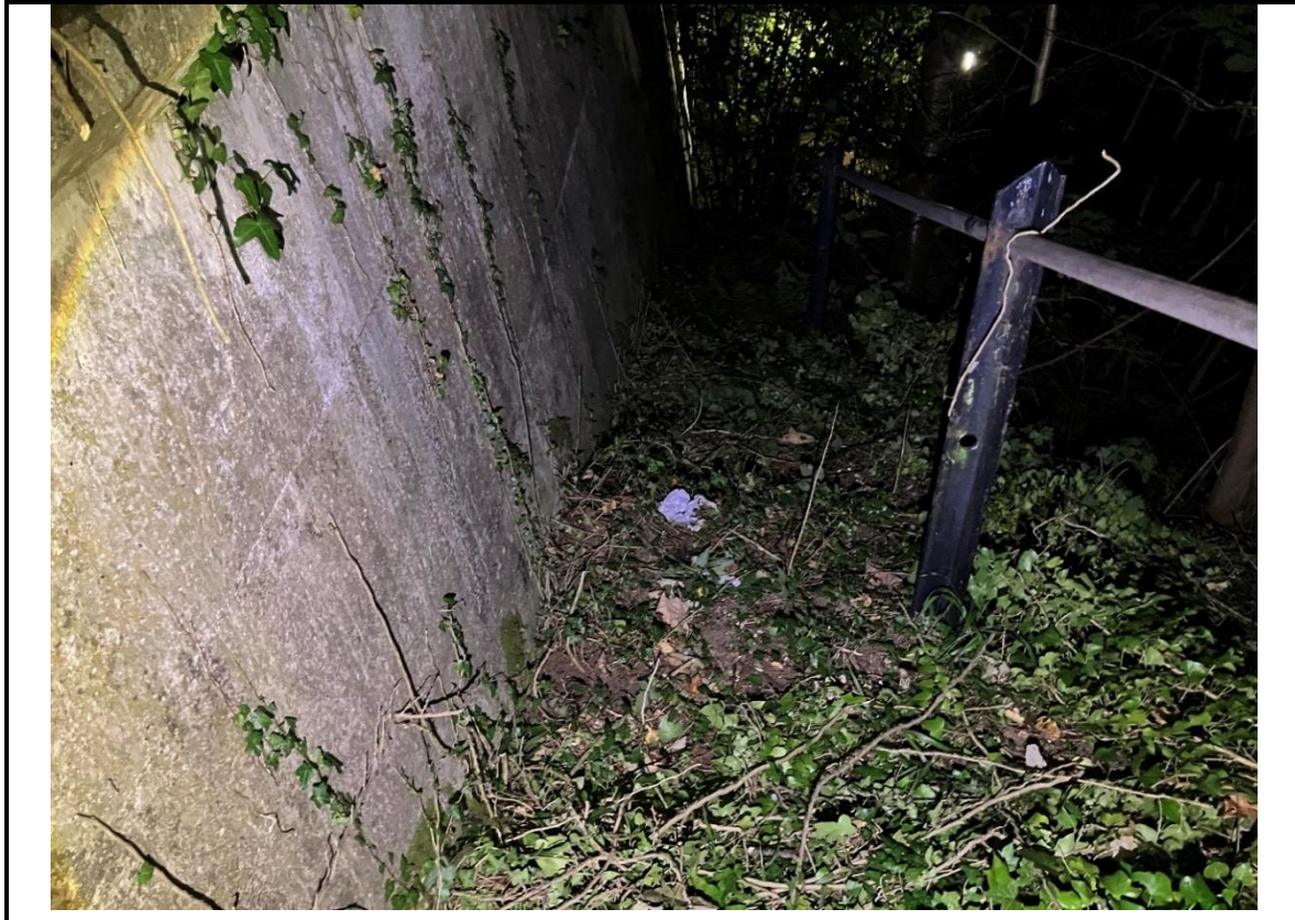
1717_P45_2024 Southwest wingwall - Leaching & vegetation growth
