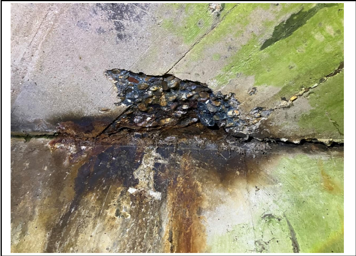
1717_P9_2024 Abutment/soffit interface - Concrete spalling
