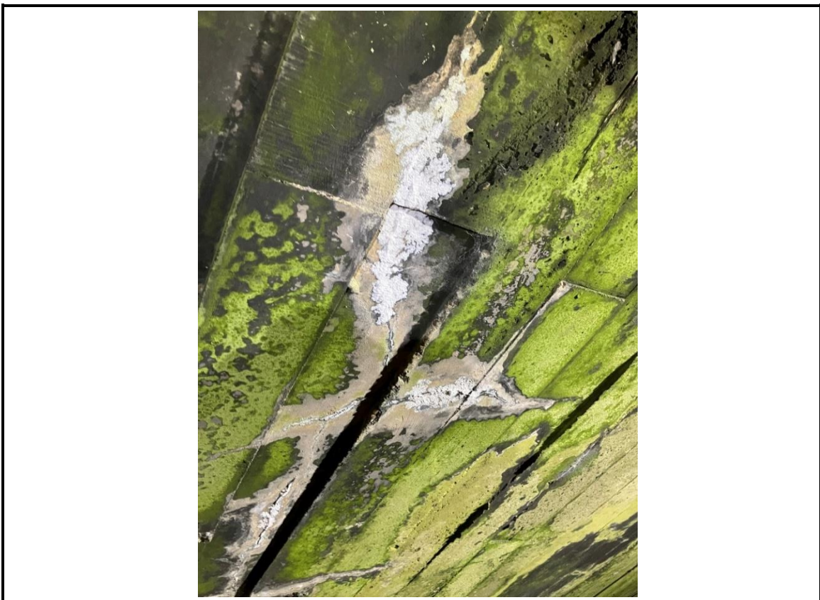
1717_P10_2024 Bridge soffit - Cracking and minor spalling
