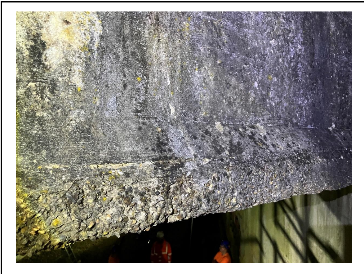
1717_P12_2024 North deck edge – Minor concrete spalling
