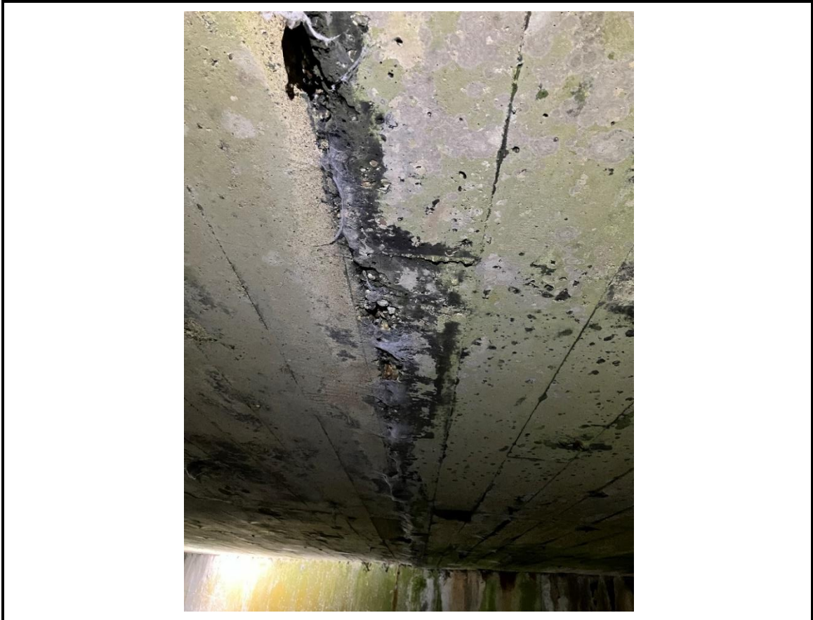
1717_P14_2024 Bridge soffit – Concrete spalling & honeycombing
