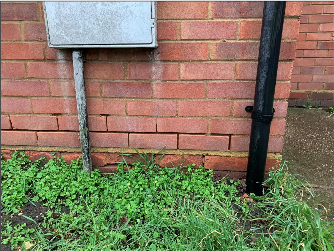
Image 4 – High water level marks post event showing erosion to brickwork
