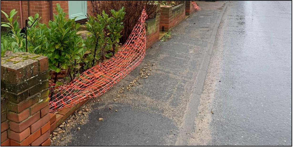
Image 5 - Post event damage
