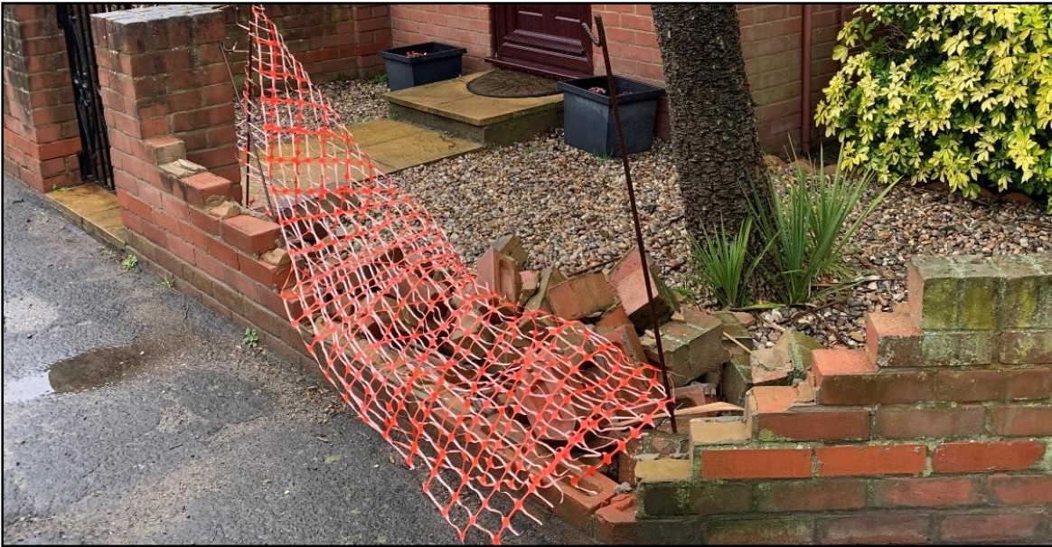
Image 7 - Post event damage
