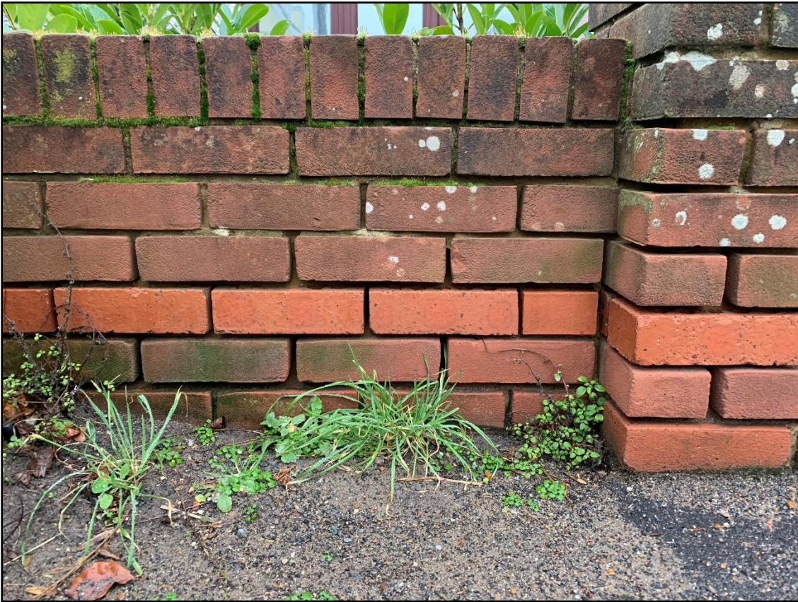
Image 6 - Post event damage
